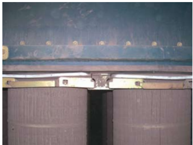
Warped mounting plates encourage gasket leaks.
