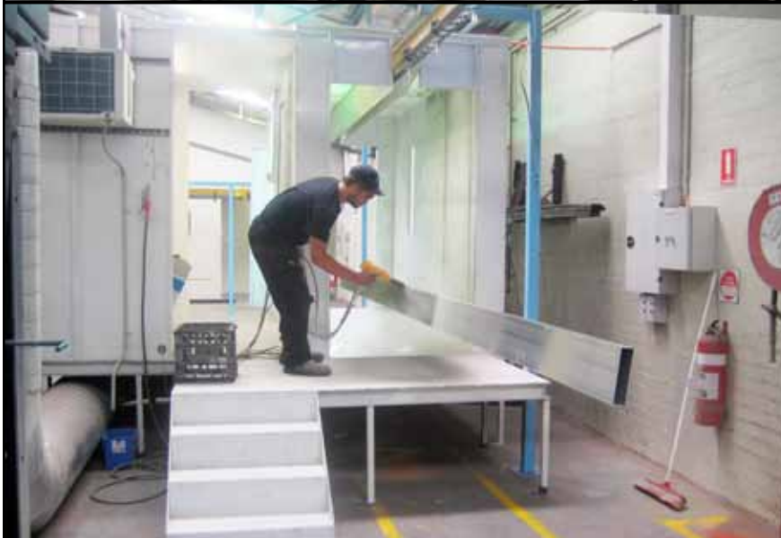
GS4 at Dolphin Coatings in Miranda, NSW on a Powder Coating Spray Paint Booth.
