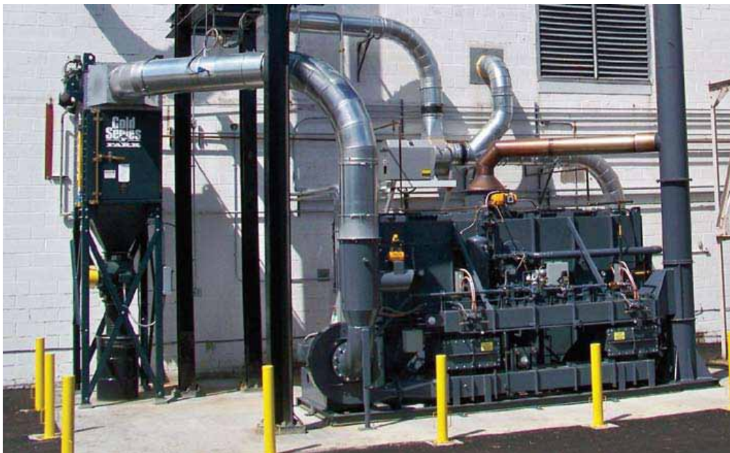
Completed GS6 unit pictured after 1 year of operation running at less than 1" of static pressure across the filters.
