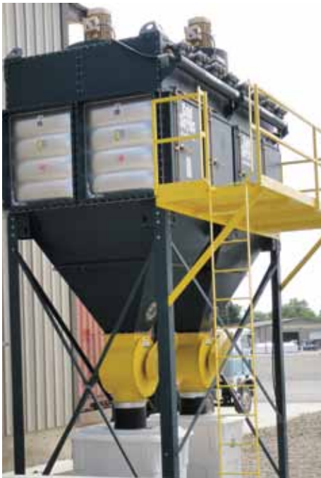
Explosion vents installed for safety.
