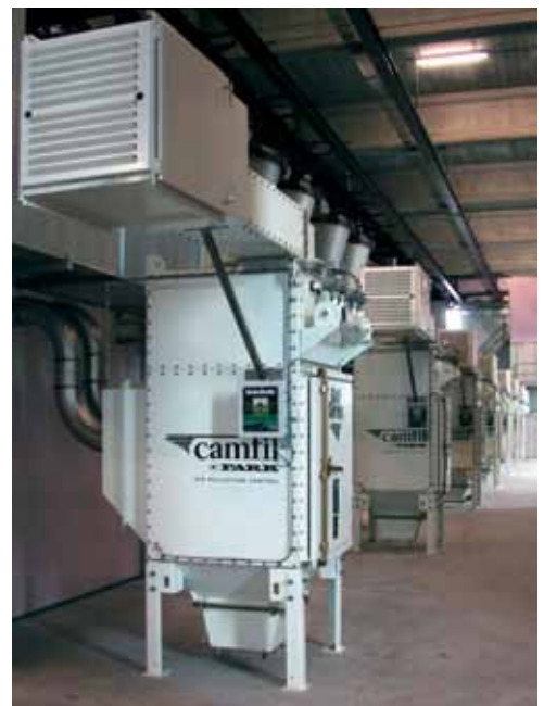
Farr Gold Series® dust collectors located at Huijbregts Group, in Helmond, The Netherlands.
