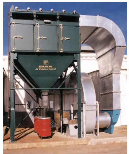
The Farr Gold Series GS36 replaced a poorly performing competitor unit.
