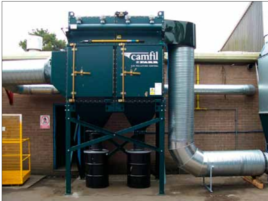
A Gold Series® GS12 dust collector located at Terrill Bros. Ltd., in Hayle, Cornwall, UK.
