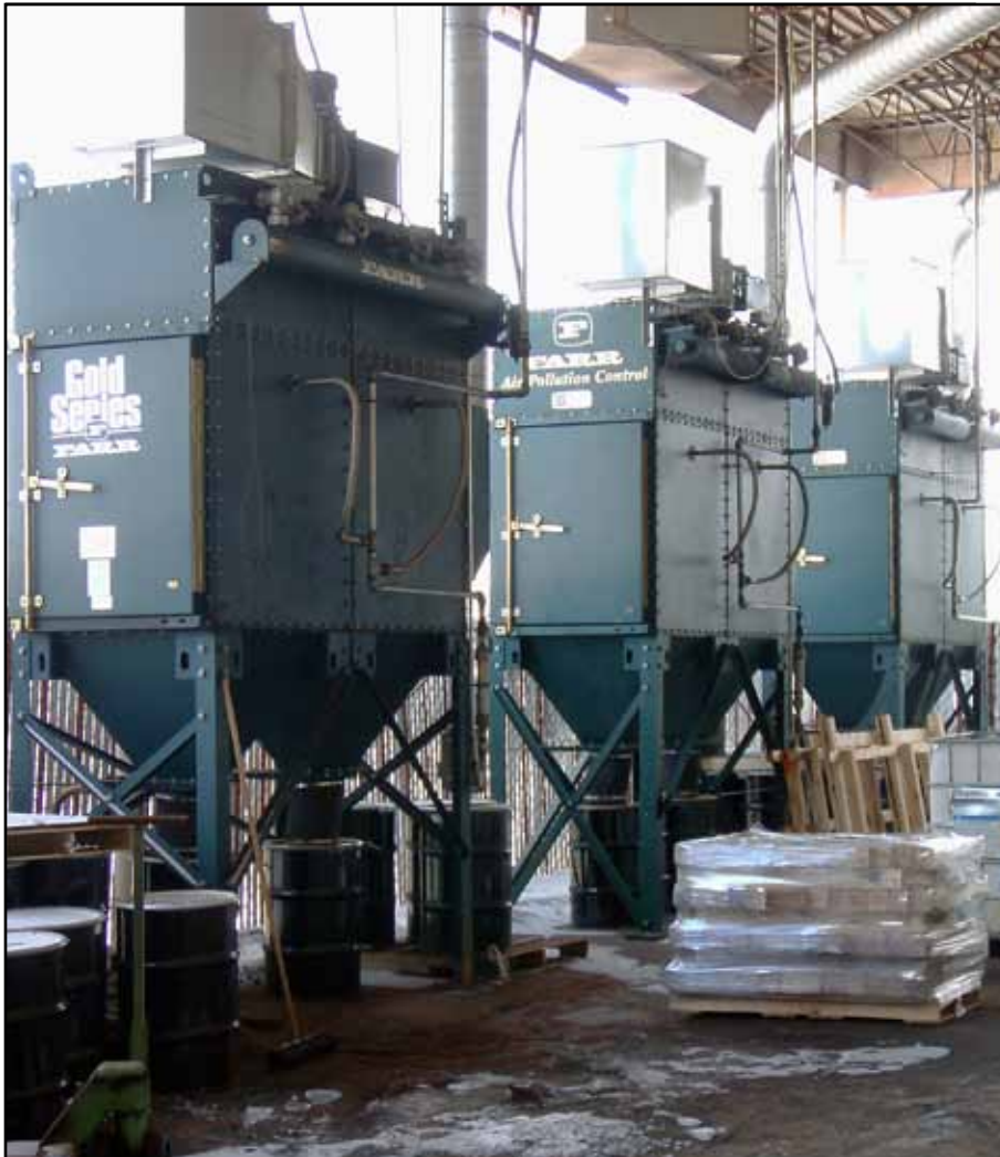
Three Gold Series GS8 Dust Collectors at Tennant Company in Minneapolis, MN.
